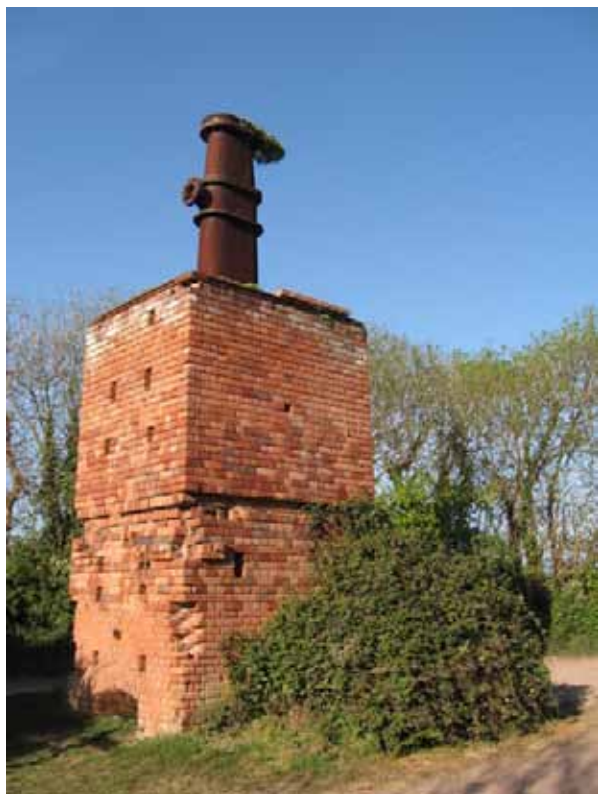
Figure 4.15 The surviving retort at Kilve, West Somerset. © Copyright Chris Andrews and licensed for reuse under the Creative Commons Licence.
